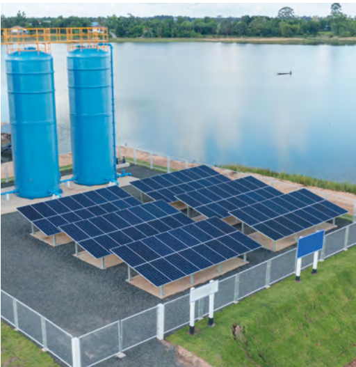
Water Pumping Systems
