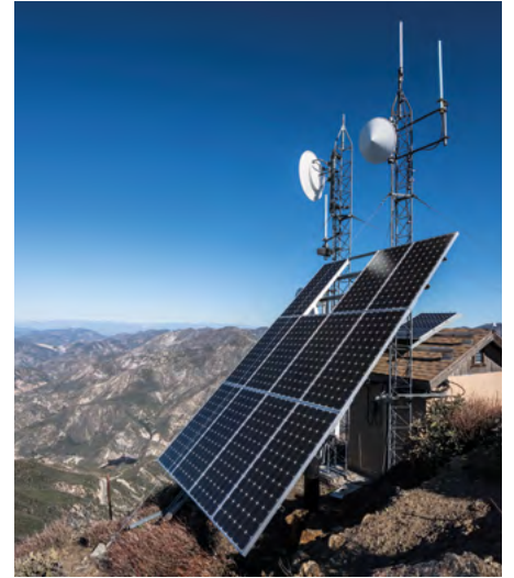
Remote Telecom Stations
